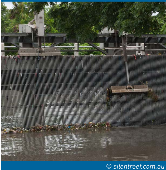
Gross pollutant trap blocks rubbish from reaching the ocean
